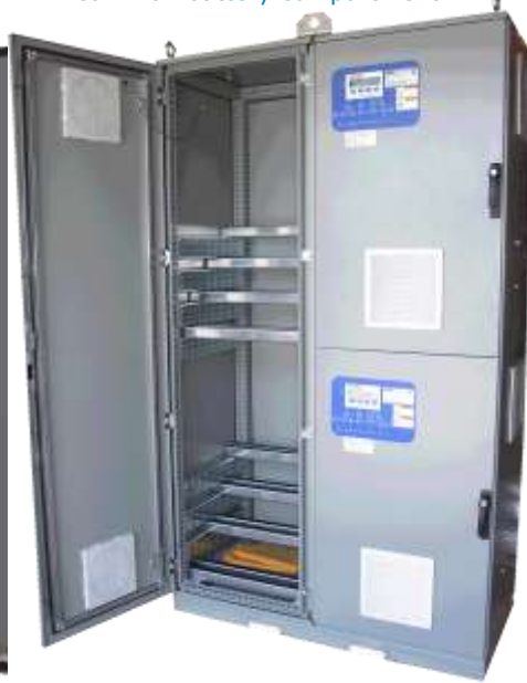
Redundant chargers with common battery compartment
